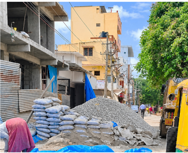
Residents of Sultan Palya Main Road, near the bus stop, are facing inconvenience as cement and jelly stones from an ongoing house construction have been dumped on the main road. The materials have spread across the road, making it difficult for pedestrians to walk and motorists to ride safely. There is also a risk of vehicles skidding, which could lead to accidents and injuries, especially when children are travelling on two-wheelers. Residents request the concerned authorities to remove the construction materials and clear the road at the earliest.
