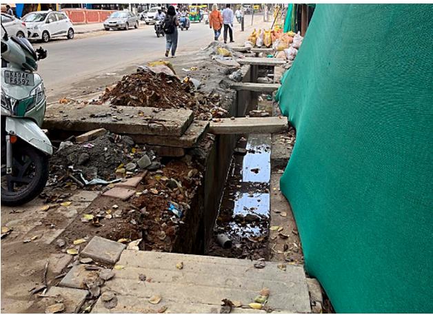
A broken footpath on Seshadripuram 1st Main Road, located behind Seshadripuram Law College, dangerously leads straight into an open gutter. Surrounded by schools, colleges, and residences, residents demand an immediate fix before a pedestrian is seriously injured in the dark.
