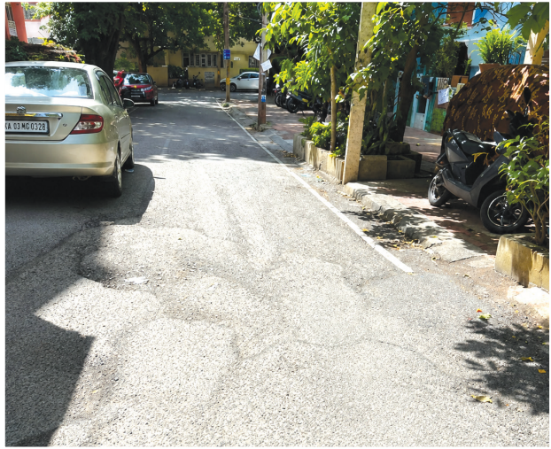
Residents along Central Street, off Serpentine Road, grapple with severely deteriorated road conditions throughout the entire residential stretch. The deeply damaged surface poses a daily safety hazard for children and senior citizens navigating the neighborhood, as well as significant risks for all commuters on the route.
