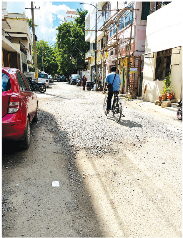
Residents along NS Iyengar Street, off Nehru Nagar Main Road, endure a persistent struggle with crumbling roads. Shoddy, short-lived patchwork collapses under regular traffic, leaving deep hazards that threaten the safety of motorists daily.
