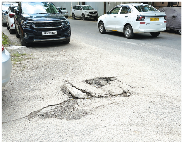
A gaping ditch near the Kumar Park dental clinic on Serpentine Road poses a daily hazard for commuters. Despite repeated complaints, authorities only apply temporary patch works. Residents demand a permanent solution to prevent severe accidents on this high-risk stretch before a tragedy occurs.
