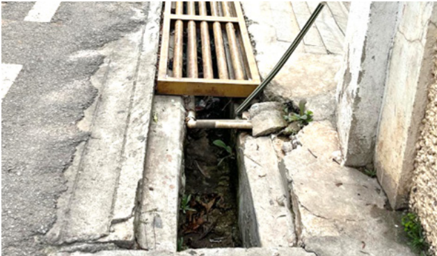
Residents of Cunningham Crescent Road have urged authorities to cover an open drainage path located almost next to the Bosch Guest House and opposite a small school. Locals warn that the unprotected hazard poses a severe injury risk to pedestrians, particularly during rain or in low-light conditions.
