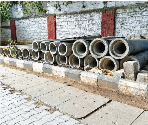
Abandoned roadwork equipment on Palace Cross Road has languished for months, turning into an open site for garbage dumping and public spitting. Residents demand to know when authorities will finally clear the abandoned machinery and relieve the neighborhood of the mounting stench and unhygienic conditions.
