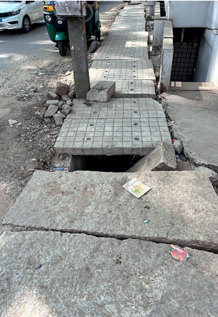
Residents of Seshadripuram 2nd Main Road warn that an unbarricaded, missing footpath slab near Hercules Tyres poses a severe hazard. Uncleared construction debris and deep gaps right at a busy vehicular turning point endanger pedestrians daily.
