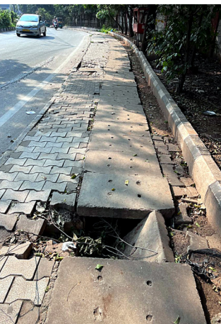
Pedestrians walking toward Bengaluru Palace along Palace Road—opposite MSI Services Private Limited—face a hazardous missing footpath slab. Compounding the danger in this high-footfall tourist and student corridor, the area lacks proper streetlights, prompting urgent calls for immediate municipal repairs.
