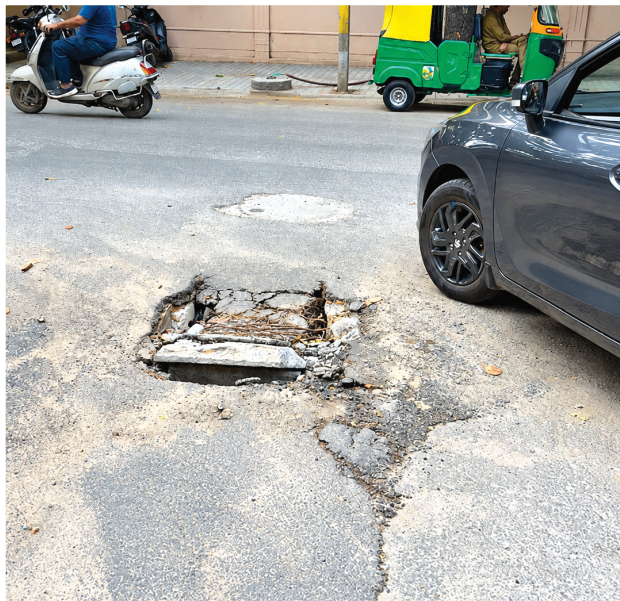
Unmarked and deeply hazardous, a massive pothole at the intersection of Serpentine Road and 7th Cross is threatening commuters. Residents report that the persistent ditch poses an immediate danger to motorists and pedestrians alike, urging municipal authorities to urgently repair the corner before a serious accident occurs.
