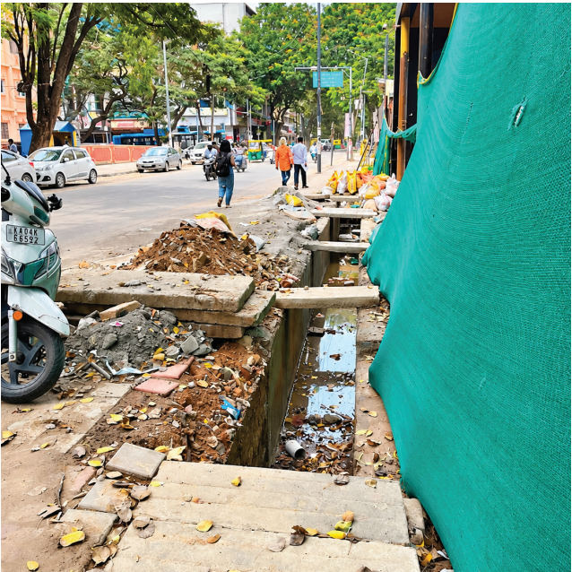
A broken footpath on Seshadripuram 1st Main Road, located behind Seshadripuram Law College, dangerously leads straight into an open gutter. Surrounded by schools, colleges, and residences, residents demand an immediate fix before a pedestrian is seriously injured in the dark.
