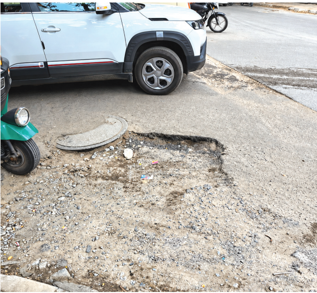
Commuters and residents near Apoorva Bakery on Seshadripuram 1st Main Road decry the hazardous link road intersection. Poor lighting and severe potholes create major crash risks, endangering pedestrians and motorists alike, especially during rain.
