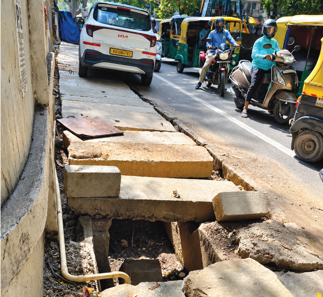
A missing section of the footpath on Palace Road, right at the corner of Hotel Tulip Inn near Vyalalikaval Circle, poses a severe hazard for pedestrians navigating the heavy traffic and nearby bus stop.
