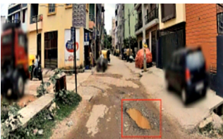
Representative pothole from the 14,393 identified across the network (Ward 20).
