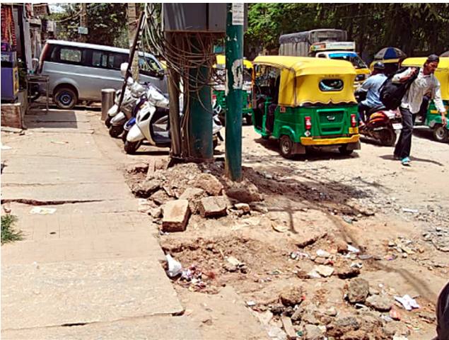
Pedestrians near Kadugondanahalli Police Station are struggling to cross the stretch safely due to the lack of proper footpaths. The area urgently needs the authorities' attention to ensure pedestrian safety.
