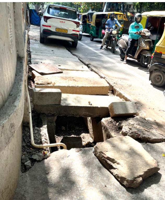
A missing section of the footpath on Palace Road, right at the corner of Hotel Tulip Inn near Vyalikaval Circle, poses a severe hazard for pedestrians navigating the heavy traffic and nearby bus stop.
