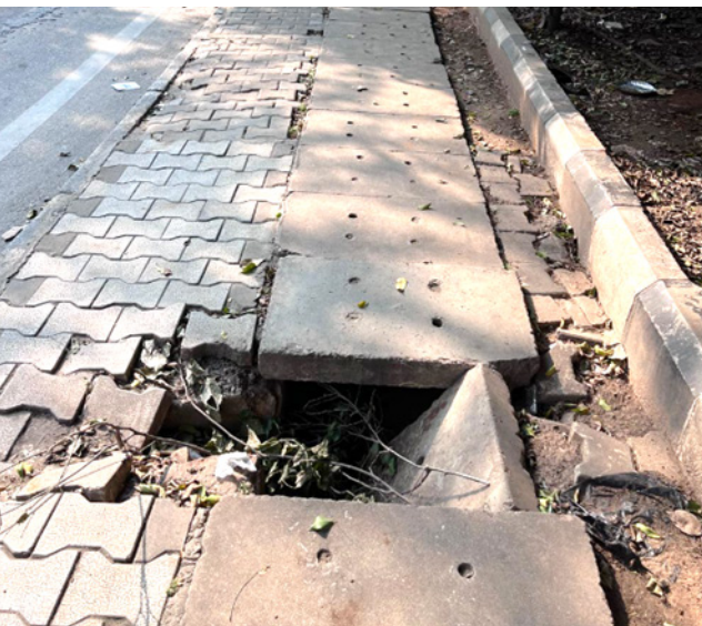
Pedestrians walking toward Bengaluru Palace along Palace Road—opposite MSI Services Private Limited—face a hazardous missing footpath slab. Compounding the danger in this high-footfall tourist and student corridor, the area lacks proper streetlights, prompting urgent calls for immediate municipal repairs.
