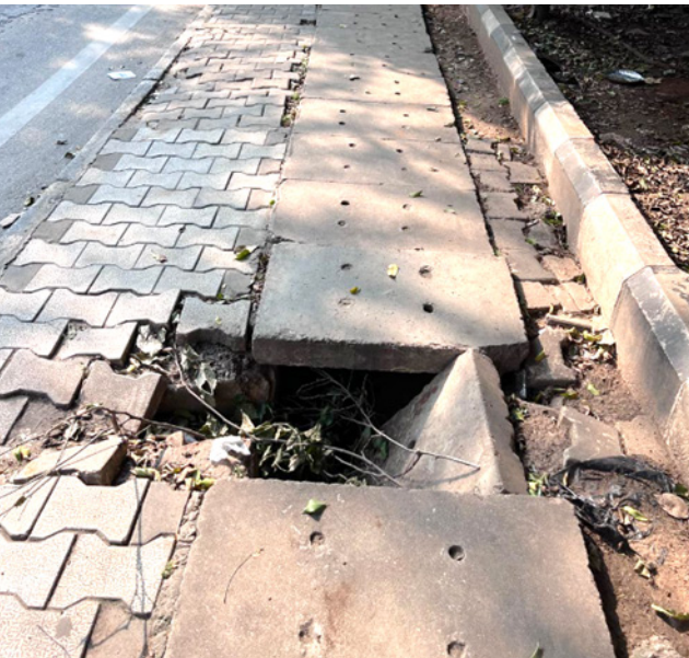
Pedestrians walking toward Bengaluru Palace along Palace Road—opposite MSI Services Private Limited—face a hazardous missing footpath slab. Compounding the danger in this high-footfall tourist and student corridor, the area lacks proper streetlights, prompting urgent calls for immediate municipal repairs.
