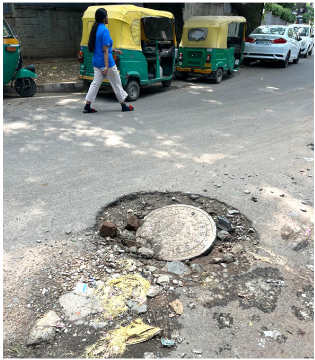
A broken drain cover on Cunningham Crescent Road, directly in front of Prestige Exotica, is surrounded by loose debris, creating a severe public hazard for pedestrians and motorists alike.
