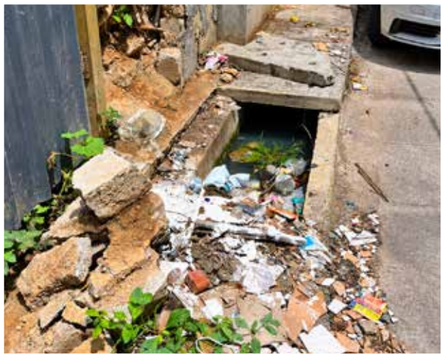
A half-open drain choked with construction debris on 1st Cross Road, Seshadripuram 1st Main Road, has become a severe public health hazard. Situated right next to the Sri Rangam Srimadh Aandavana Ashram, the clogged drain serves as a dangerous breeding ground for disease-bearing vectors. Local residents warn that the unattended filth poses an imminent threat to the heavy footfall of devotees and families visiting the area daily, demanding urgent intervention from civic authorities.
