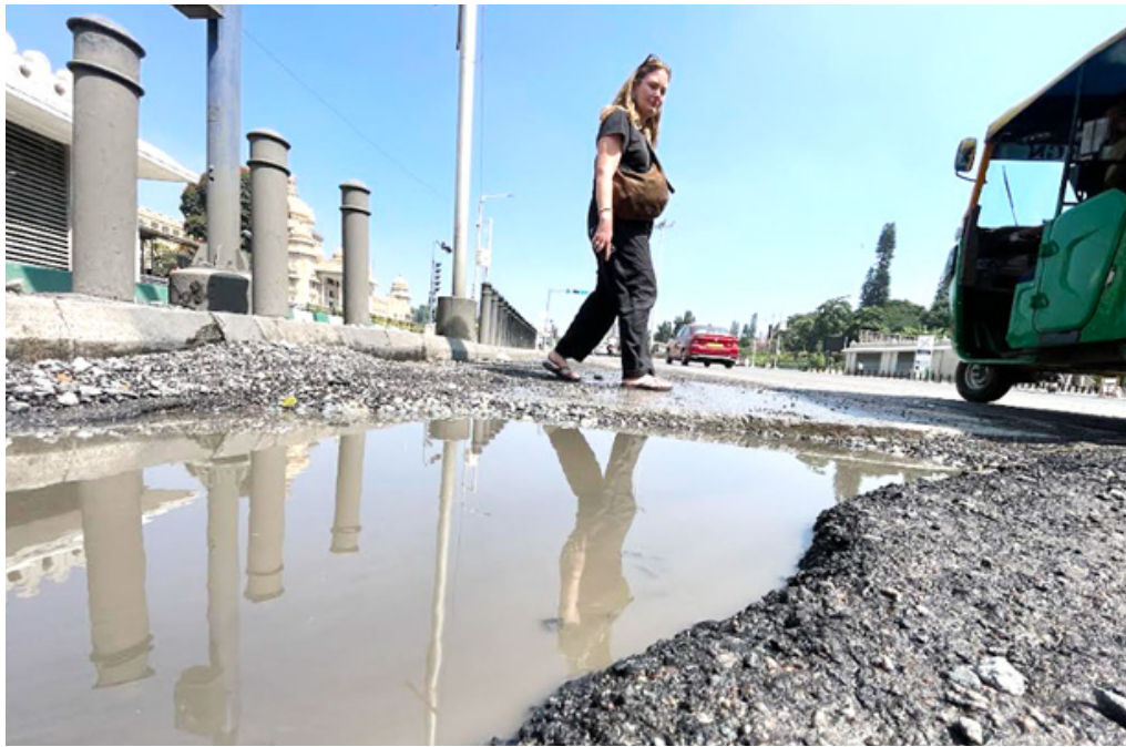
A foreign woman strolls along a severely damaged road adjacent to Shantaveri Gopalgowda Circle on Ambedkar Veedhi, near Vidhana Soudha, in Bengaluru on Thursday.
