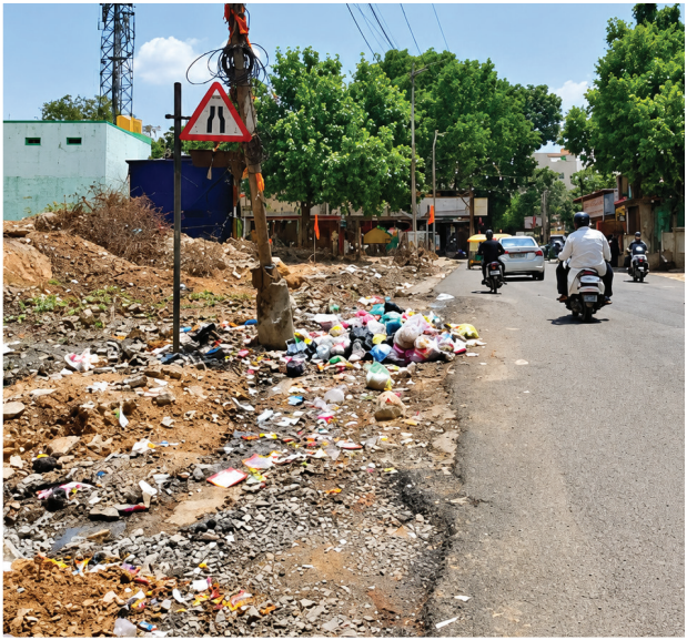
The incomplete road work near KG Halli (near Arabic College) is now being misused as a garbage dumping spot. Piles are spilling onto the main thoroughfare, causing foul odor, health risks, and traffic disruptions. Requesting local authorities to clear the waste immediately and expedite road completion.
