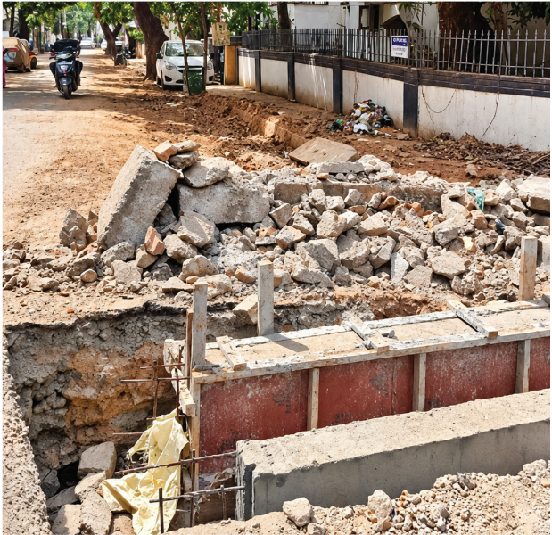
Construction materials, stones, and heavy debris have spilled over onto the roadside near Hutchins Road, narrowing the path, generating severe dust nuisance, and risking vehicle/pedestrian safety. Requesting authorities to clear the debris and enforce site cleanup.
