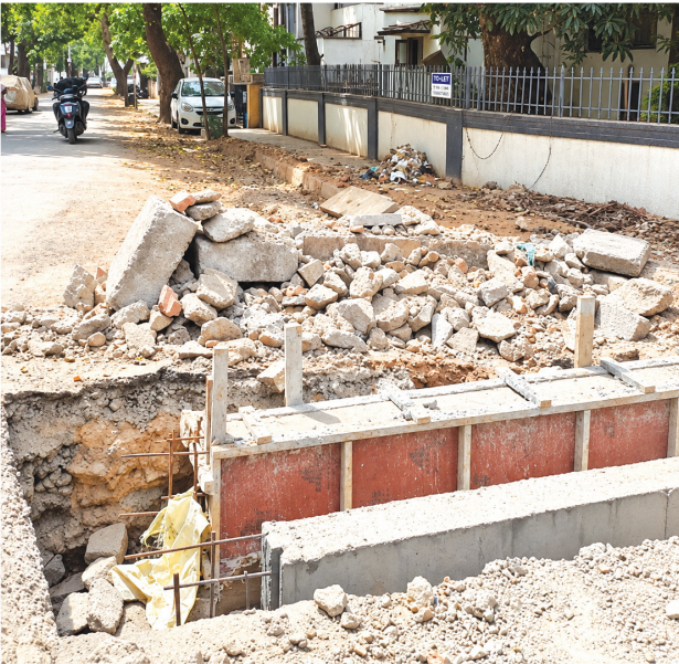
Construction materials, stones, and heavy debris have spilled over onto the roadside near Hutchins Road, narrowing the path, generating severe dust nuisance, and risking vehicle/pedestrian safety. Requesting authorities to clear the debris and enforce site cleanup
