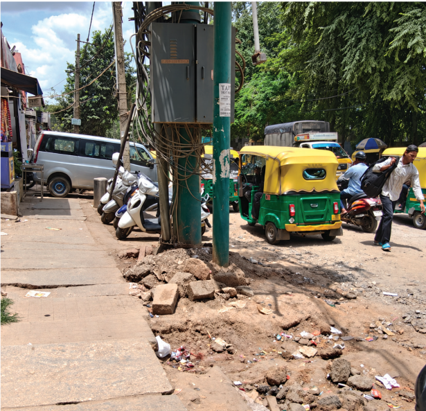
Pedestrians near Kadugondanahalli Police Station are struggling to cross the stretch safely due to the lack of proper footpaths. The area urgently needs the authorities' attention to ensure pedestrian safety.
