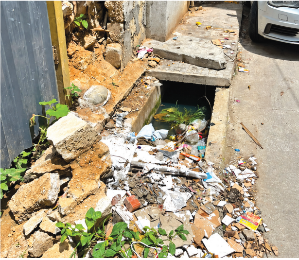
A half-open drain choked with construction debris on 1st Cross Road, Seshadripuram 1st Main Road, has become a severe public health hazard. Situated right next to the Sri Rangam Srimadh Aandavana Ashram, the clogged drain serves as a dangerous breeding ground for disease-bearing vectors. Local residents warn that the unattended filth poses an imminent threat to the heavy footfall of devotees and families visiting the area daily, demanding urgent intervention from civic authorities.
