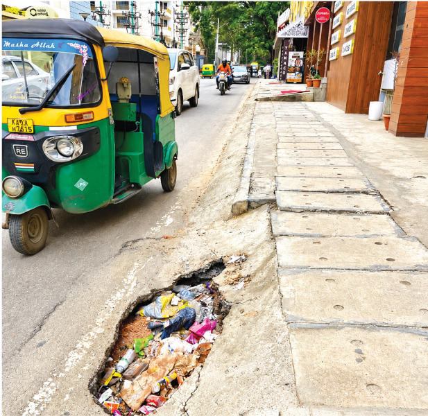
A dangerous ditch spanning both the footpath and the road near Tawazo Café on 6th Main Road, AK Colony, Mathikere Extension, poses a major hazard to students and residents. Citizens urge municipal authorities to fix this critical safety risk immediately.
