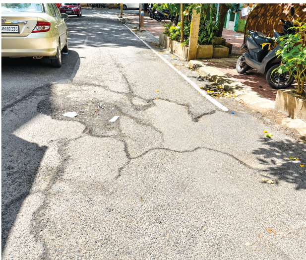
Residents along Central Street, off Serpentine Road, grapple with severely deteriorated road conditions throughout the entire residential stretch. The deeply damaged surface poses a daily safety hazard for children and senior citizens navigating the neighborhood, as well as significant risks for all commuters on the route.
