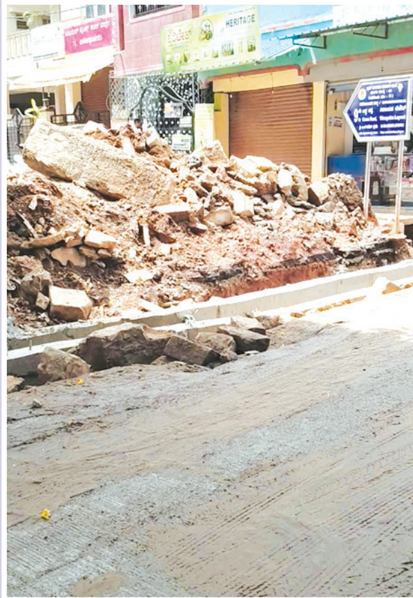
Residents of Vinayaka Layout, 9th Cross, near Manoranayapalya Main Road, are facing severe inconvenience due to a road blockage in the area which has been underwork from past 3 weeks. Residents have urged the concerned authorities to take action and clear the obstruction to restore smooth traffic movement.
