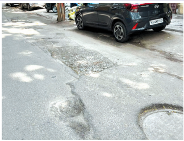
Pedestrians and travelers who use the Vasanth Nagar 11th main road ( near Imperial Hotel ) have been reporting on the unsafe roads with a lot of potholes. Irrespective of any type of complaints, the respected governance body would patch it up, but the patch would turn into a pothole in no time.
