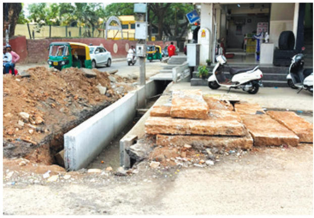
Pedestrians and residents living on the link road ( Seshadripuram ) stretch face extreme difficulty due to the very slow progress of the drain works. The drainage work being left open without any type of barricade pose as an extremely dangerous threat. Enormous amount of dust is leaving the senior citizens and children with breathing issues.
