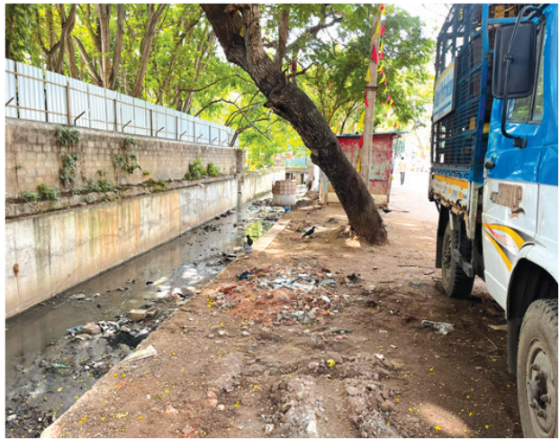
Open, unprotected, unmarked drain on the Jasma Devi Bhavan Road. Has no barrier or at least a notice or fencing is calling for a mishap to take place. Residents and travelers say that this poses as a huge risk as it is pitch dark at night and surprisingly it is right next to the KPCC office (Queens road).
