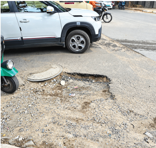
Commuters and residents near Apoorva Bakery on Seshadripuram 1st Main Road decry the hazardous link road intersection. Poor lighting and severe potholes create major crash risks, endangering pedestrians and motorists alike, especially during rain.
