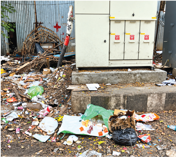
An illegal garbage dump on North Park Road right next to the Seshadripuram Post Office creates a severe public health hazard. Plagued by an unbearable stench, the polluted spot sits right beside a BBMP washroom, two temples, a swimming pool, an indoor stadium, and Seshadripuram Composite College, prompting urgent student demands for a permanent fix.
