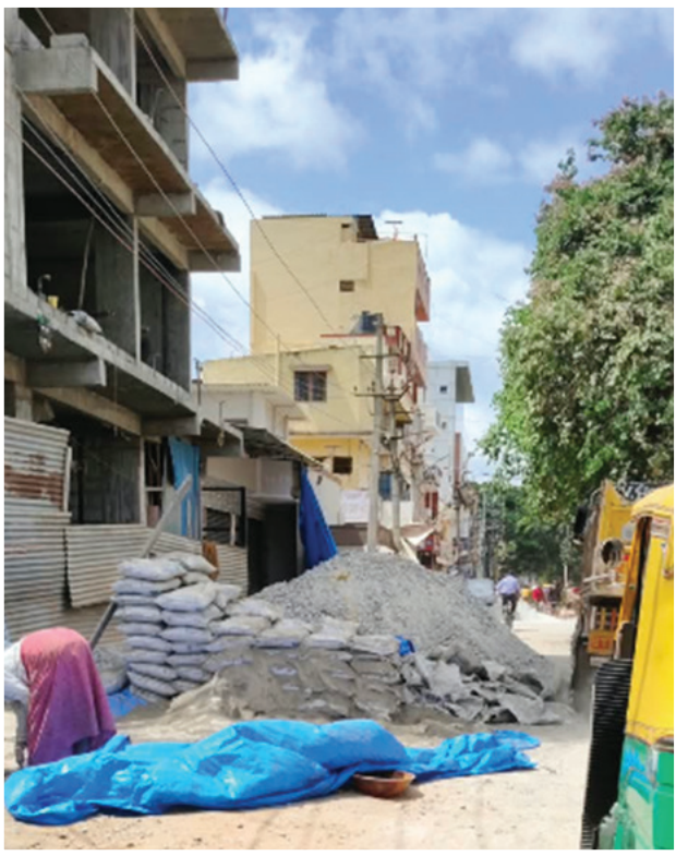
Residents near the Sultanpalya Main Road bus stop are facing severe inconvenience after cement and jelly stones from an ongoing house construction were dumped directly onto the thoroughfare. The scattered materials have blocked walkways for pedestrians and created treacherous riding conditions for motorists. This blockage poses a high risk of vehicle skidding and potential accidents, particularly endangering children traveling on two-wheelers.
