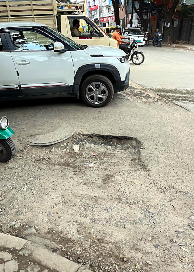
Commuters and residents near Apoorva Bakery on Seshadripuram 1st Main Road decry the hazardous link road intersection. Poor lighting and severe potholes create major crash risks, endangering pedestrians and motorists alike, especially during rain.
