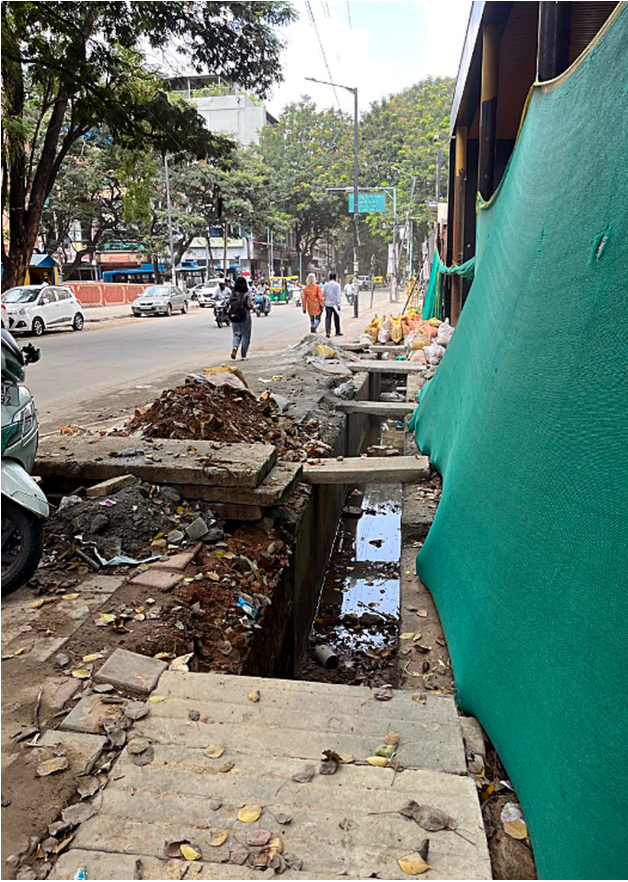
A broken footpath on Seshadripuram 1st Main Road, located behind Seshadripuram Law College, dangerously leads straight into an open gutter. Surrounded by schools, colleges, and residences, residents demand an immediate fix before a pedestrian is seriously injured in the dark.
