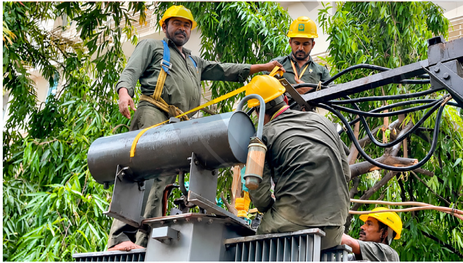
Power utility workers at a transformer.
