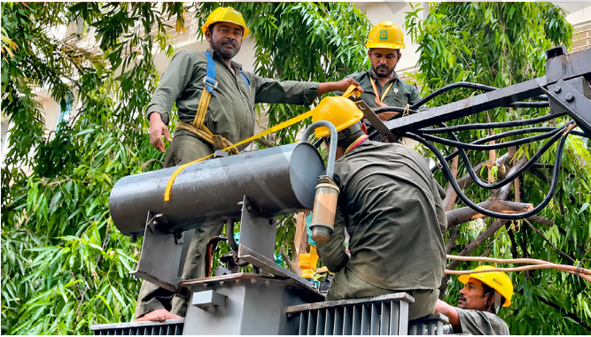
Power utility workers at a transformer.
