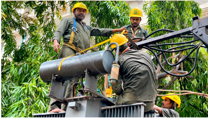
Power utility workers at a transformer.
